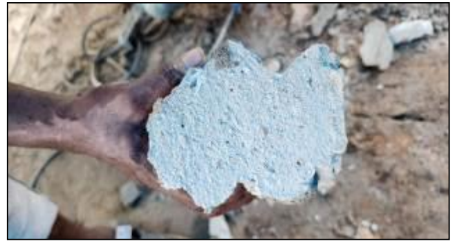
Fig -45: Cross section examination. No serious cold joints, shrinkage cracks or voids found, chance of porosity
