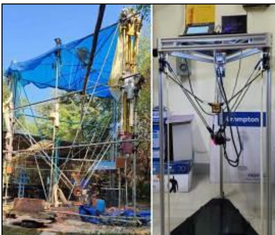
Fig -8: Delta 3D printer at CUSAT, Kochi & Delta 3D concrete printer at Minvayu, Auroville
