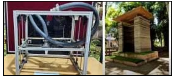
Fig -3: India’s 1 st 3d Concrete printer at IIT Madras & India’s 1 st 3d Concrete printed structure at IIT Madras
