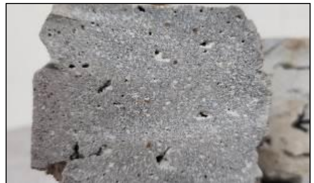
Fig -32: Enlarged view of core sample cross section: Strong and hard surface texture found. No serious issues with inter layer bonding.
