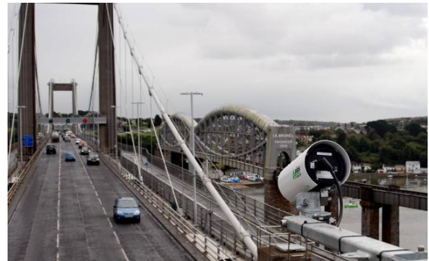
Fig.5. ALPR system installed on a bridge
