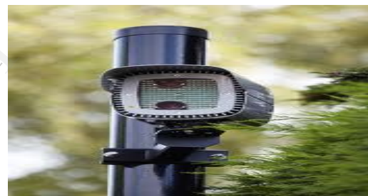
Fig.6. An ALPR system installed on a pole
