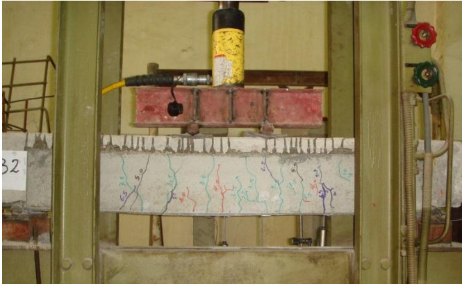
Fig. 9. Crack patterns of specimen B2 strengthened with external additional horizontal steel bars 2Ø8 with 2 vertical steel clamps.
