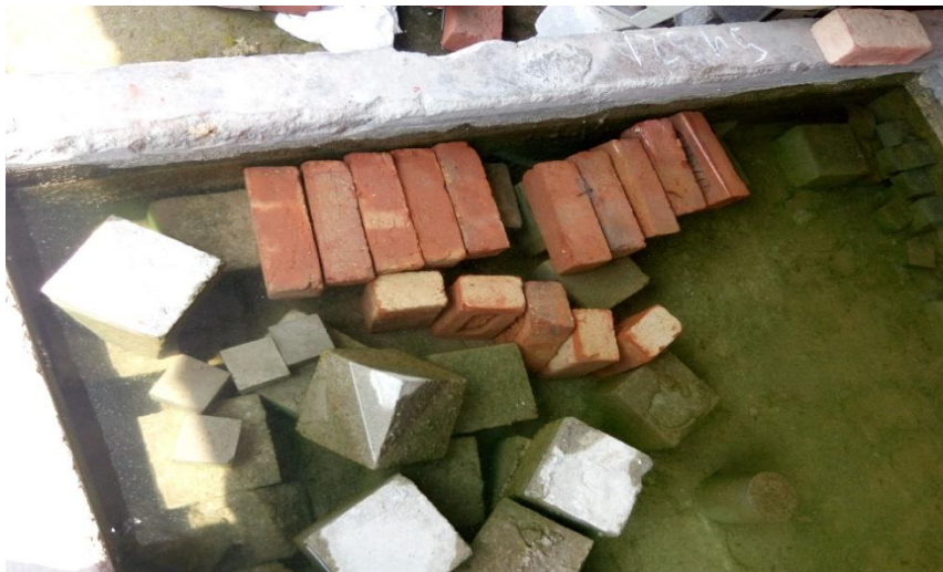
Figure 2. Water absorption tank
