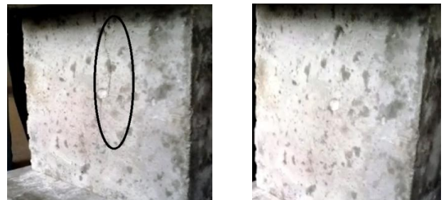
Figure 4: Crack healed concrete specimen With crack (left) & Healed Specimen (right)
