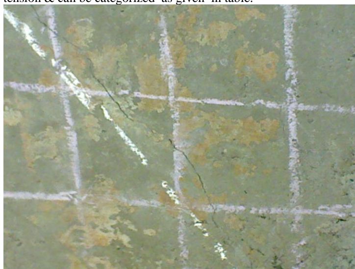
Image 8 Diagonal cracking in deep beam
