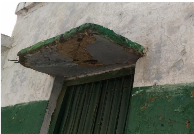
Figure 3:- Cracked Hanging Slab
