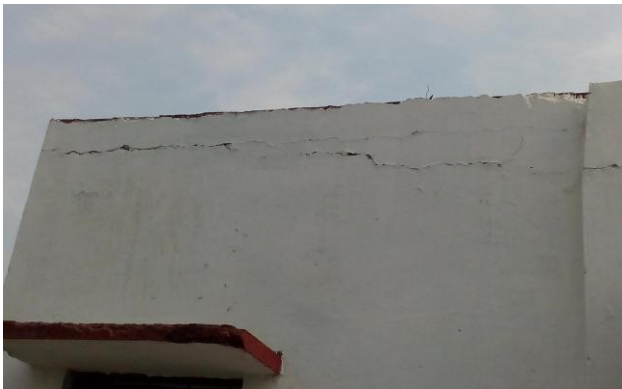
Figure 2:- Roof Wall Crack Visible
