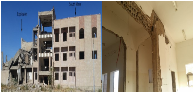
Fig. 13. General view of damaged building in Hamdan (South mass)
