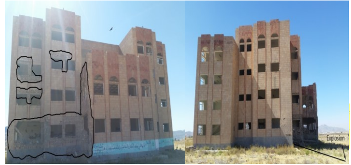
Fig. 11. General view of damaged building and Location of the explosion.
