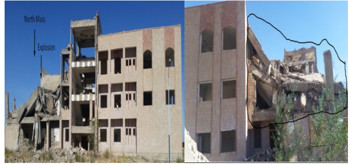
Fig. 19. General view of damaged building in Hamdan
