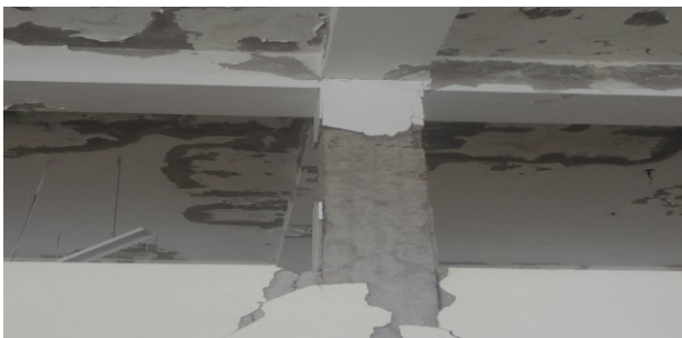
Fig. 3. Scaling in concrete column.
