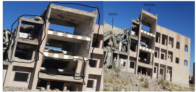
Fig. 16. General view of damaged building in Juhana
