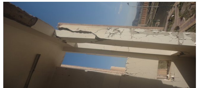
Fig. 5. Separation in concrete column
