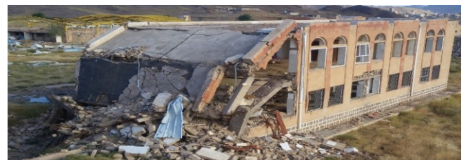
Fig. 7. Partial collapse in R.C structure
