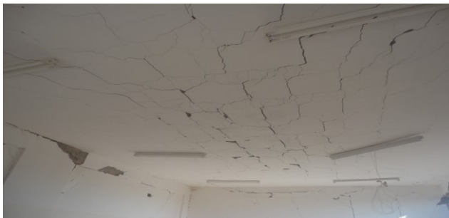
Fig. 2. Plastic deformation with cracks in concrete slab.
