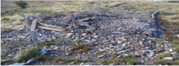
Fig. 8. Total collapse in R.C structure
