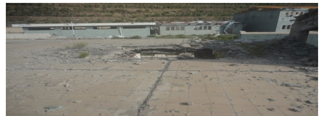
Fig. 6. Hole in concrete slab
