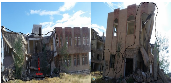
Fig. 14. General view of damaged building in Juhana
