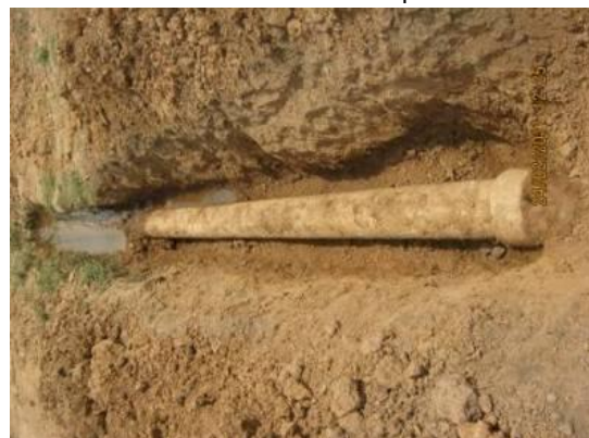
Figure 2: Broken DN200mm AC sewer close to the old waste stabilization pond
