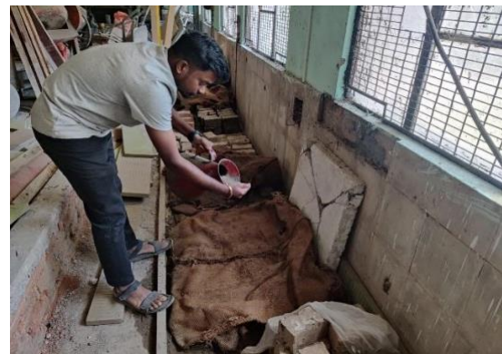
Figure 4: Curing of SSA blocks by covering with wet gunny bags for period of 28 days.
