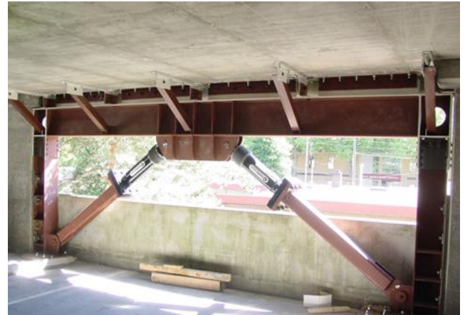
Fig 7 Provision of damper in building
