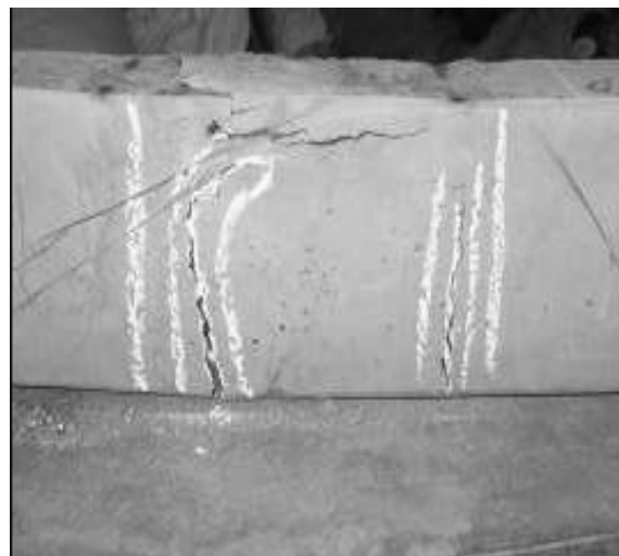
Fig 8. Crack pattern in beam reinforced with plain round bars with straight axis.
