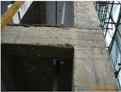
(a) Damage of beam
