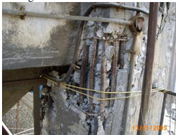
(b) Damage of column
