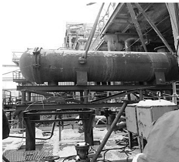
Fig. 19: Installation of metal structures of rails (a) Pipe racks (b) Rail support rack
