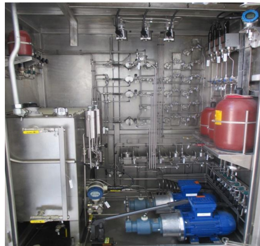
Fig.3. Well head control panel
