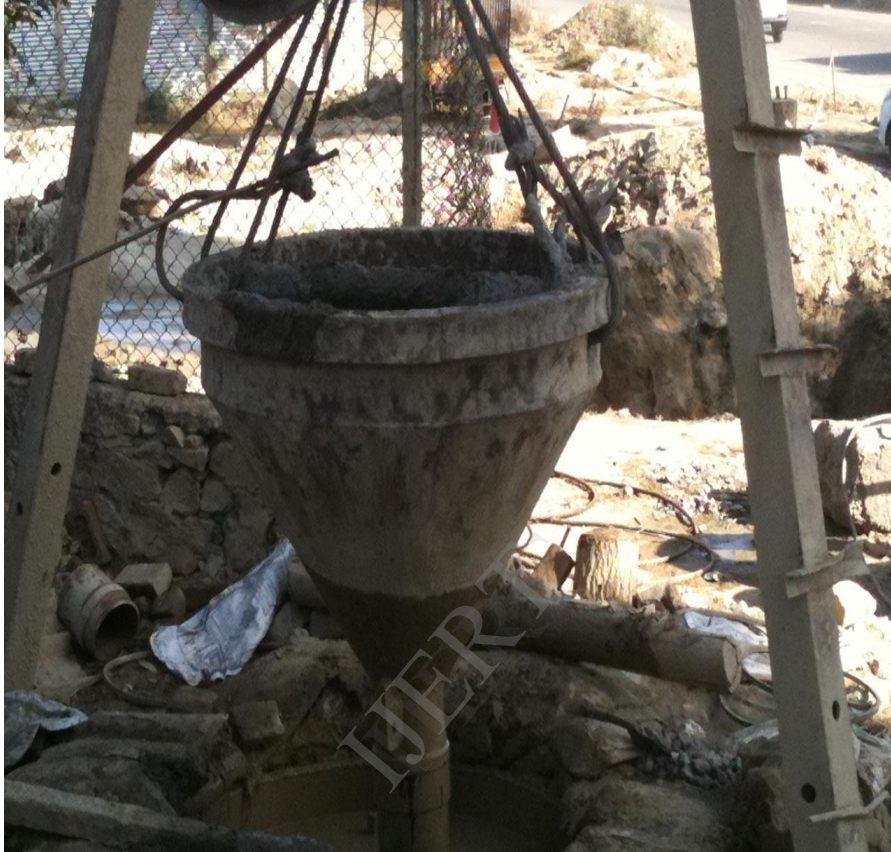
A funnel connected with a tremie pipe used for pouring concrete into the pile
