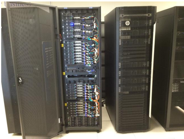
Figure 5 Prairie View A&M University IBM HPC cluster
