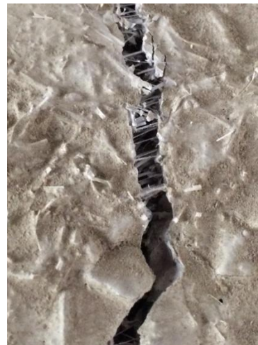
Fig. 6 Zoomed Photo of Crack Width
