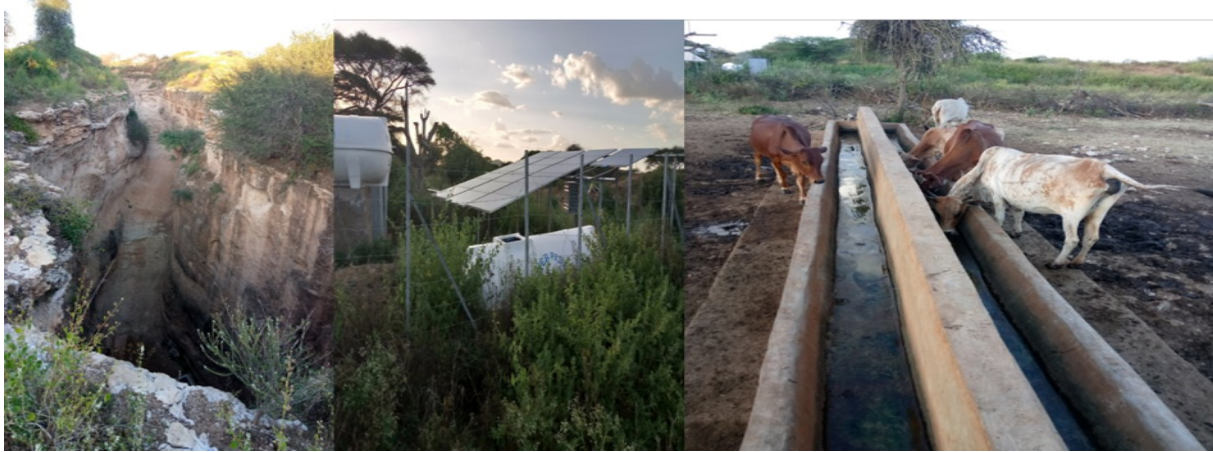
Figure 6 Solar radiation pump installed at the Gaadulticha well in Dhas
