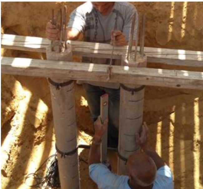
Fig. [13] Vertical Alignment of the Pile for Group (2) – Group of Two Piles
