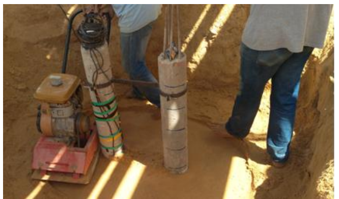
Fig. [11] Placing Soil around Tested Pile for group (2) – Group of Two Piles
