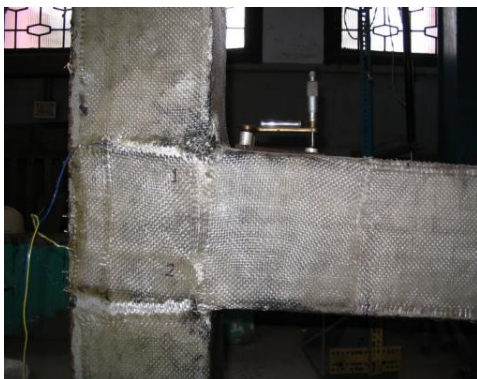
Fig. 17: Rupture of GFRP at joint
