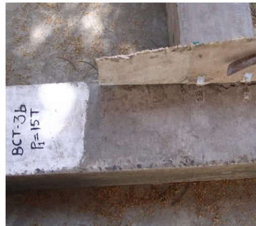
Fig. 18: De-lamination of GFRP
