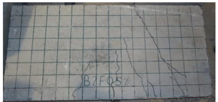
Fig 7 Crack Pattern of beam D40 AR80 [F0.5%]
