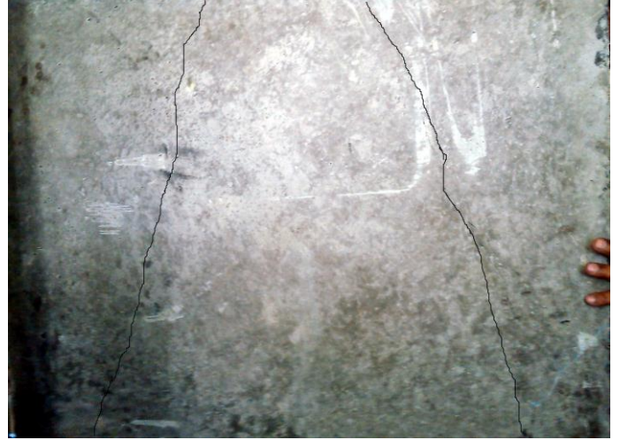
Fig 12 Crack Pattern of beam D60 AR80 [F0.75%]
