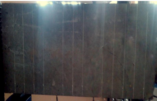
Fig 11 Crack Pattern of beam D60 AR80 [F0.5%]
