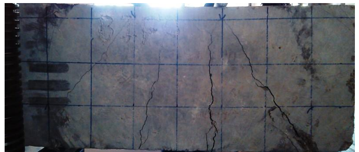
Fig 14 Crack Pattern of beam D30 NRC [F0%]
