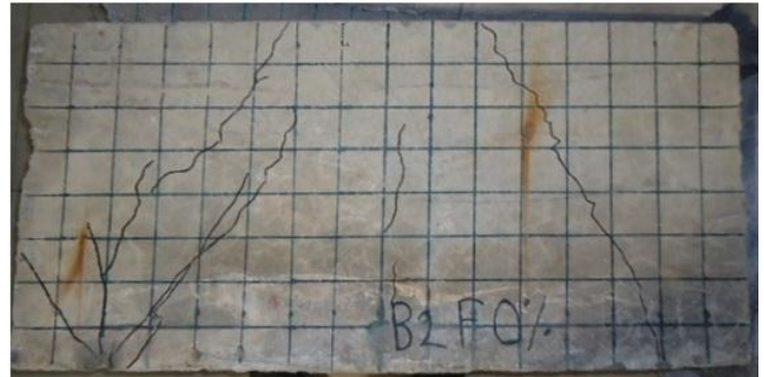
Fig 6 Crack Pattern of beam D40 NRC [F0%]
