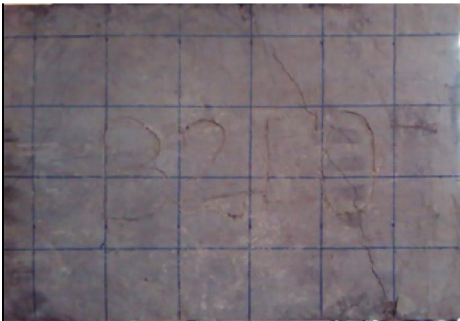
Fig 18 Crack Pattern of beam D40 NRC [F2%]
