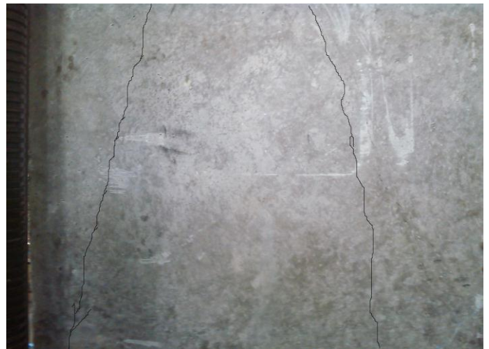
Fig 13 Crack Pattern of beam D60 AR80 [F1%]
