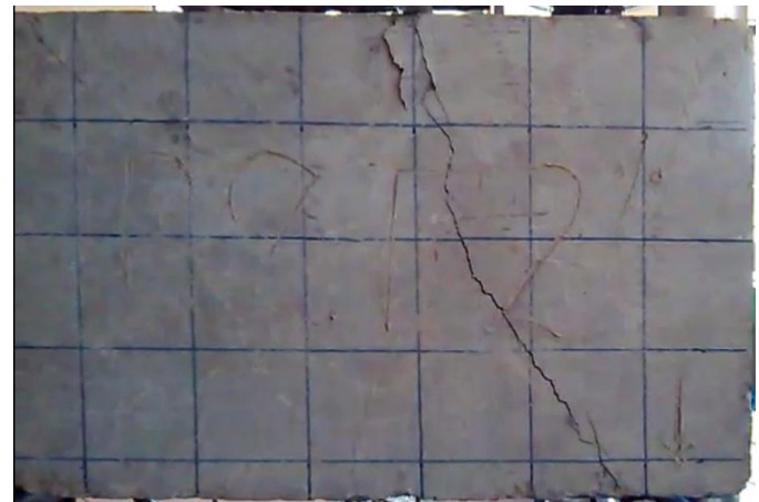
Fig 21 Crack Pattern of beam D40 AR50 [F2%]
