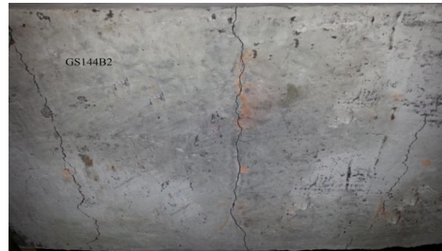
Fig 6: Failure Pattern in Geopolymer Concrete Slabs.
