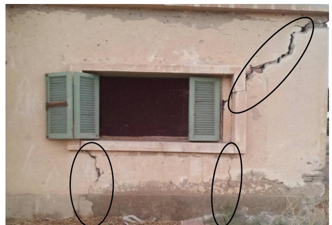
Fig. 1 Diagonal cracks over lintel and vertical cracks below window opening (Old building in elhagar city, El.fayoum) .
