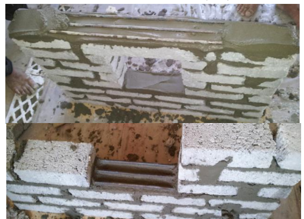
Fig. 7. Strengthening brick walls with opening using 3Ø8 steel bars embedded into bed joint mortar above lintel and sill with length (L1 = 50 cm)
