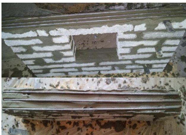
Fig. 9. Strengthening brick walls with opening using 3Ø8 steel bars embedded into bed joint mortar above lintel and sill with length (L2 = 85 cm)
