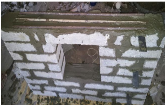
Fig. 5. Strengthening brick walls with opening using 3Ø8 steel bars embedded into bed joint mortar above lintel only with length (L2 = 65 cm)
