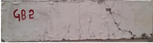
Plate 3.failure pattern of 40% GGBS with 1% SF beam
