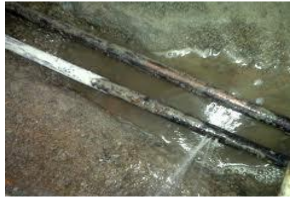
Fig. A.5(Poor material condition)
