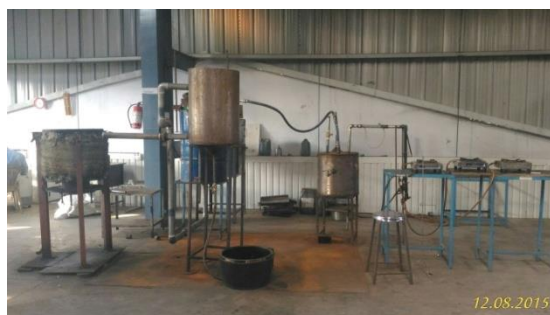
Fig.2.1: Overall assembly at plant location.
