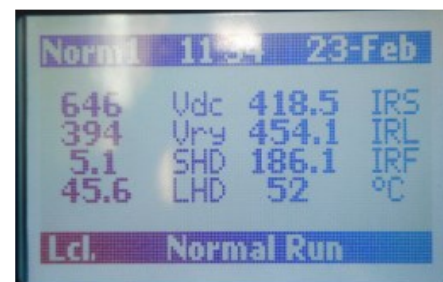
Fig 7.6 b SOURCE HARMONIC DISTORTION – 5.1 % at 93 % AHF RATING (186.1 A)
