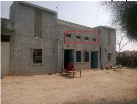
Fig. 8. Ventilator above the door openings[19]
