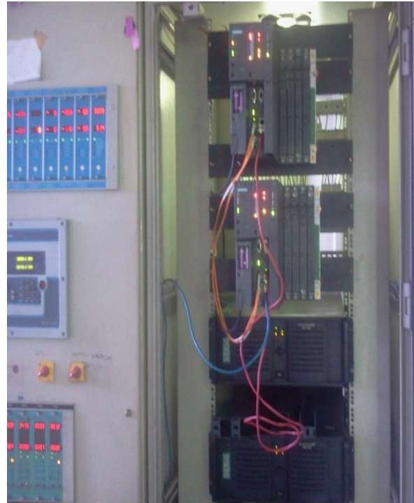
Fig. 3. Actual view of both the controllers, Above two are New Programmed PLC and Below two are DCS.
