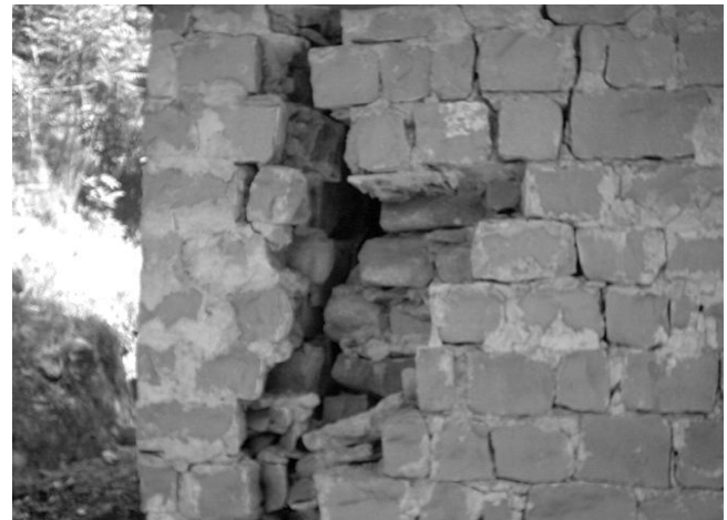
Figure 4: Typical corner joint failure of a house in earthquake
