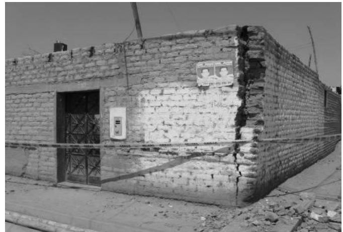
Figure 3: Corner joint failure of bonded masonry in earthquake
