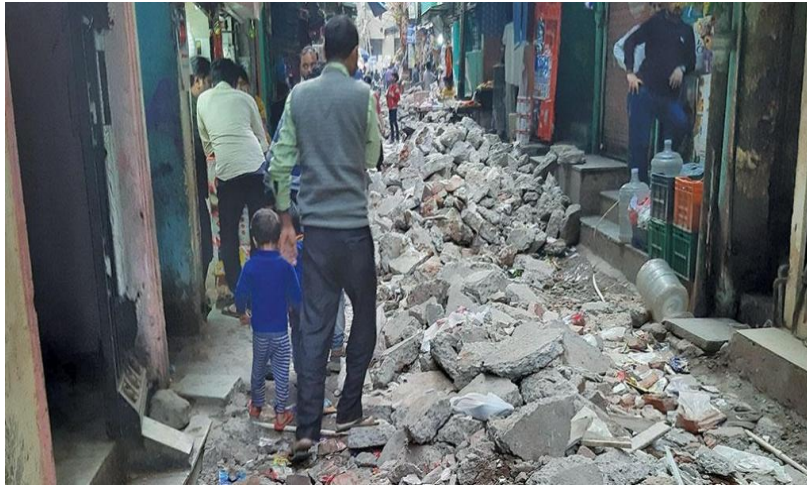
Figure: Demolition waste from a road being redeveloped in Delhi's Zamrudpur village has left no space for people even to walk. Photo: Avikal Somvanshi/CSE
