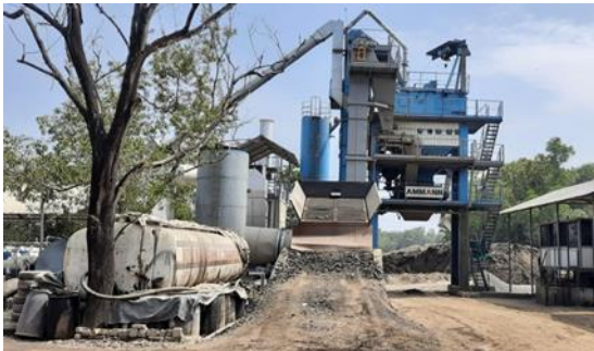
Fig No: 4 HM Plant
