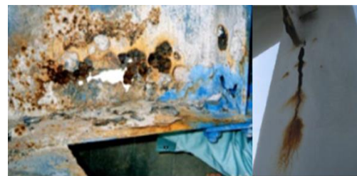
Fig. 1. Localized penetration corrosion.
