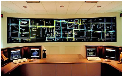
Fig. 3. Central Control Room
