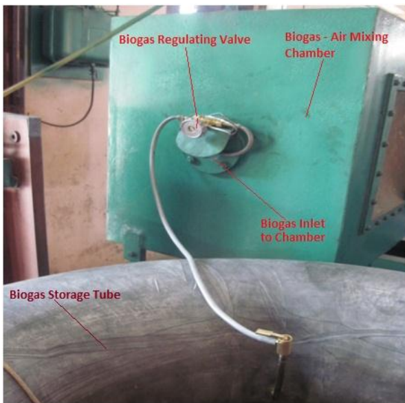
Fig 2: Experimental Arrangement with biogas storage in rubber tube
