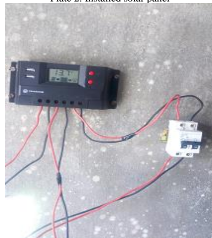
Plate 3 Installed PWM charge controller with Switch box
