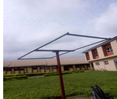
Plate 1. (a) The mounting rod in the concrete hole (b) The Mounting frame attached to the rod
