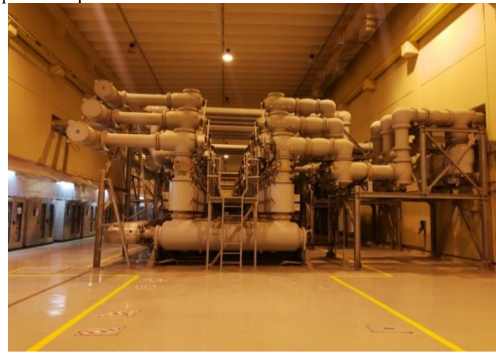
Fig (1): A typical 380kV GIS with one & half breaker scheme
