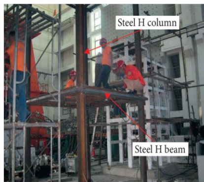
Fig. 10. The steel frame composed of steel H beams and steel H columns.
