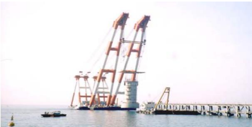
Figure 2: View of offshore concrete structure with skirt foundation just before skirt penetration. (Saito et. al., 2003)
