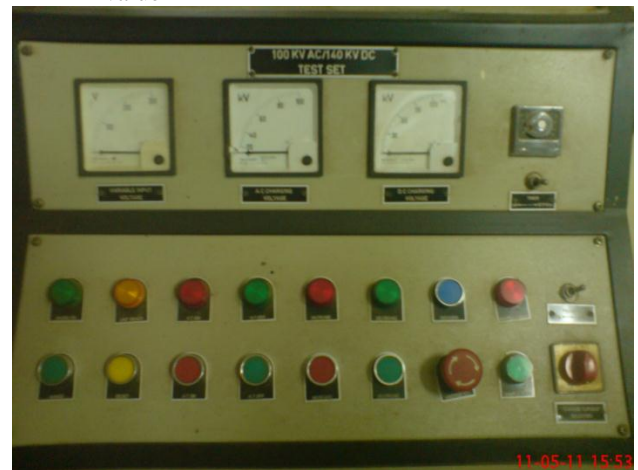
Figure.4. Control panel in the High Voltage laboratory
