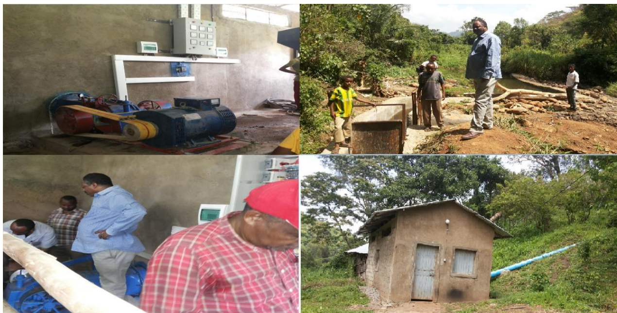
Figure .2 Internal and External part of Leku site Micro hydropower plant
