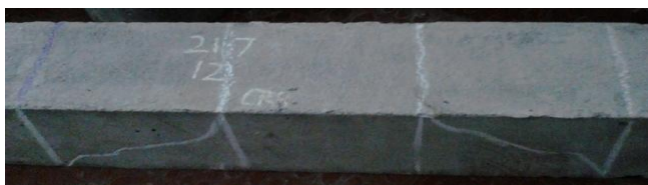
Fig. 5 Crack pattern of reinforced beam
