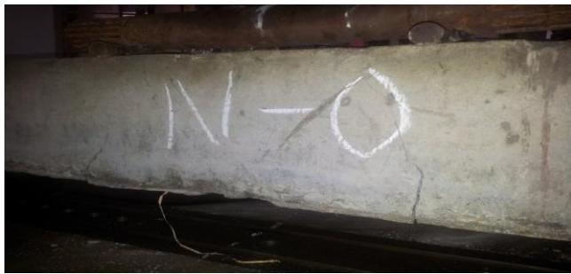
Figure8: Failure of beam NSB1
