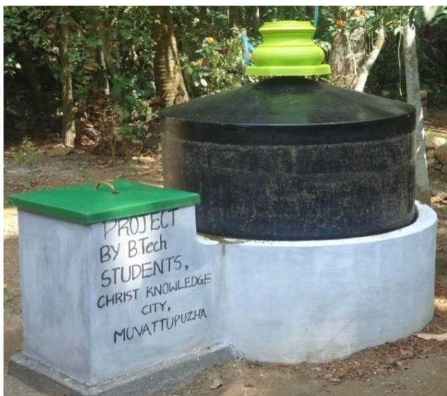
Fig.1. Bio gas plant
