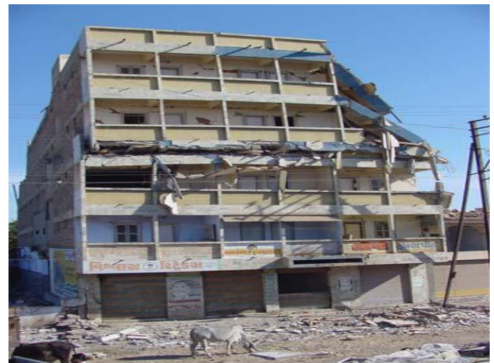
Figure 1: Collapse of soft middle storey in building at Bhuj during Bhuj Earthquake, 2001 [8]
