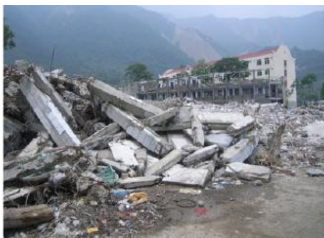
Figure 4: Complete collapse of soft storey building at Yingxiu Town of Wenchuan County during Wenchuan Earthquake, 2008 [2]
