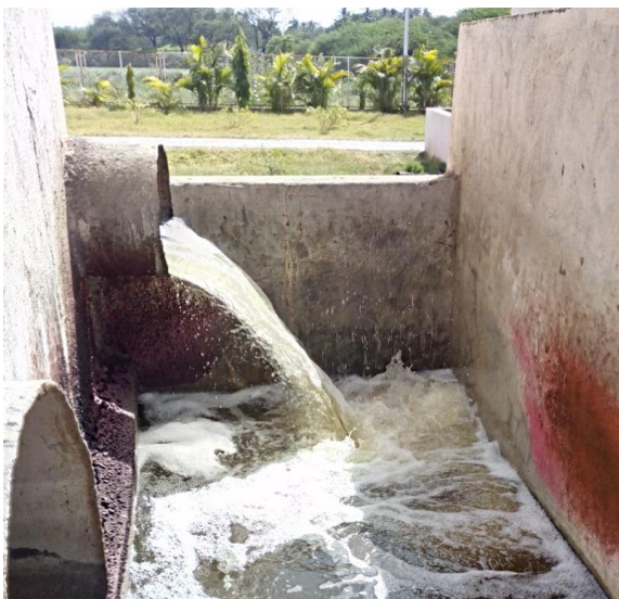
Fig. 5. Outlet of SBR reactor
