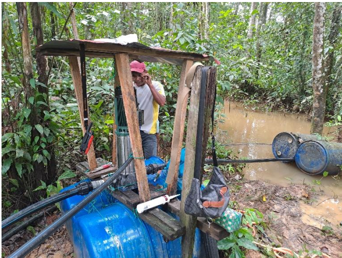
Fig. 4: On the right are the two holding tanks joined together, under which is the intake one-way valve. On the left is the 4 HP pump also on two floats.
