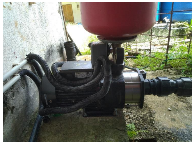
Fig. 15: The outgoing 4 HP pump to pump water from the 9000L holding tank to each home of the village
