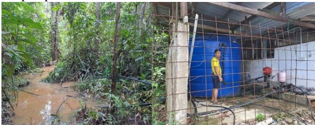
Fig. 5: The right image is the pathway back to the Pump House. On the right is the HDPE pipe carrying the 3 \Phi wires of 2.5mm 2 each. Below it is the \Phi=2'' pipe carrying the water. The other pipes are not used. The right image shows the Pump House where the 9000L holding tank, the red Pressure Tank, the left for the incoming and the right is above the outgoing 4HP pump (black color)
