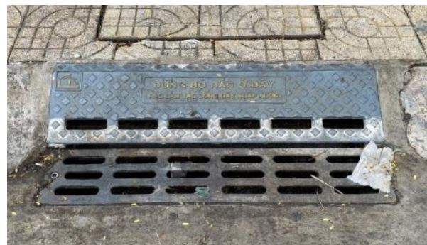
Fig. 1. Improved drainage inlet
