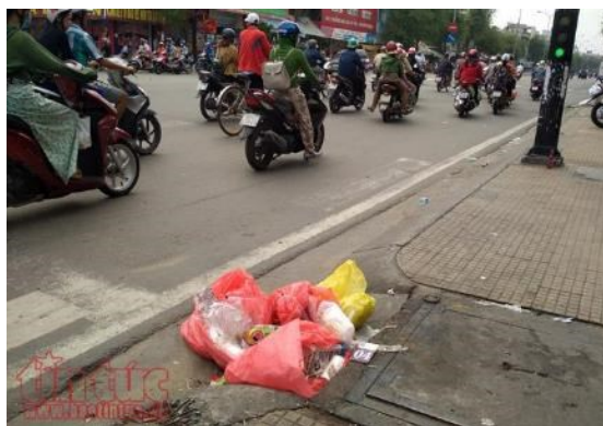
Fig. 2. Debris blocking drainage inlet (8)
