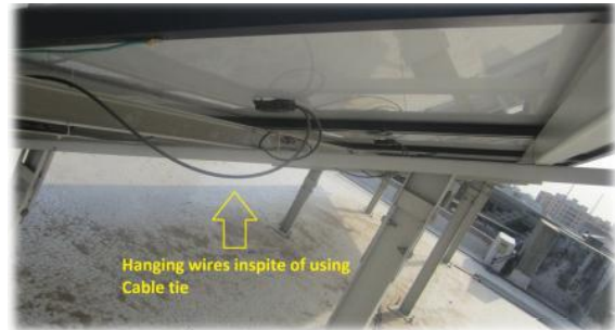
Figure 2 Wires hanging down the module
