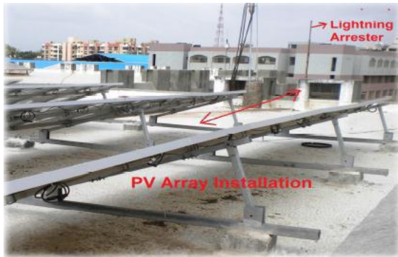
Figure 3 Position of lightning arrester
